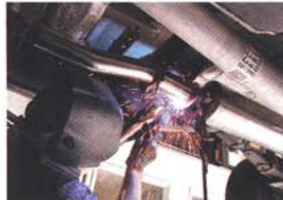
JBA welds all tubing connections for a secure installation.
